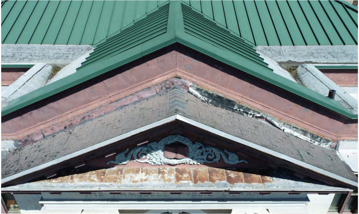
Failing roofing at pediment and cornice
