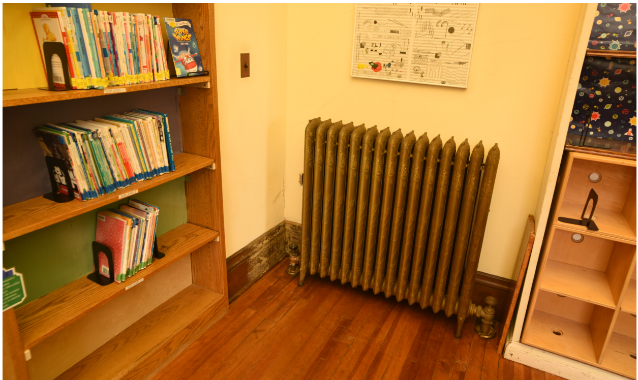
Water damage at Children's Room
