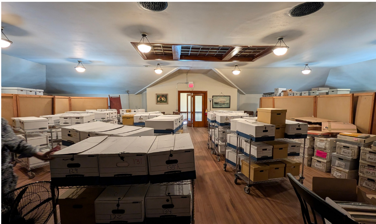
Lack of accessibility and inadequate egress to Second Floor precludes use of Great Hall
