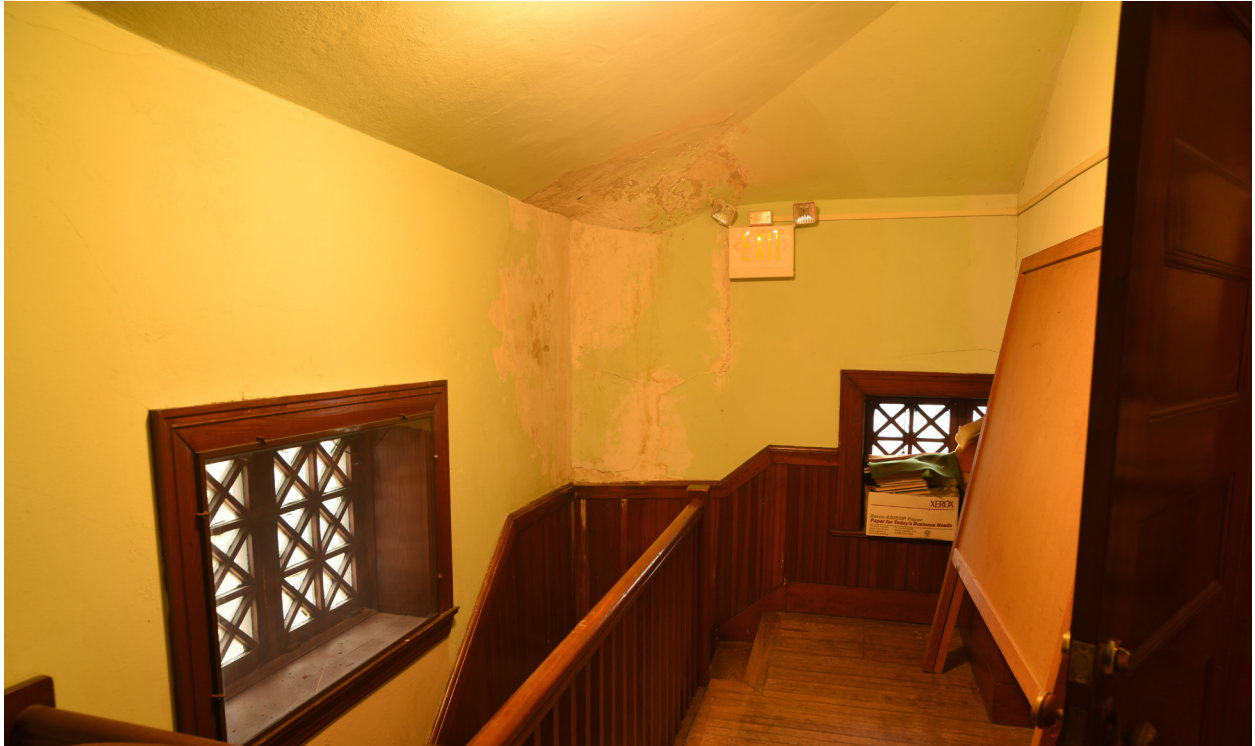
Water damage and cracked plaster at Second Floor
