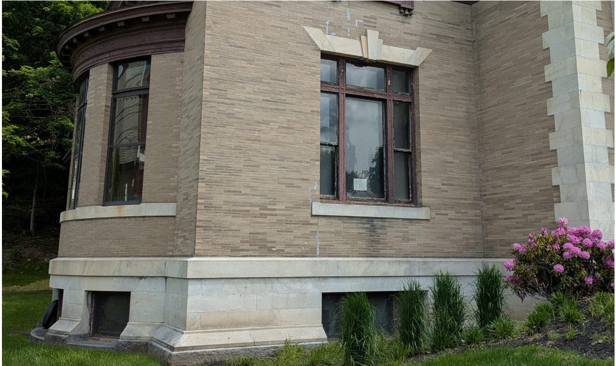
Masonry cracks and staining
