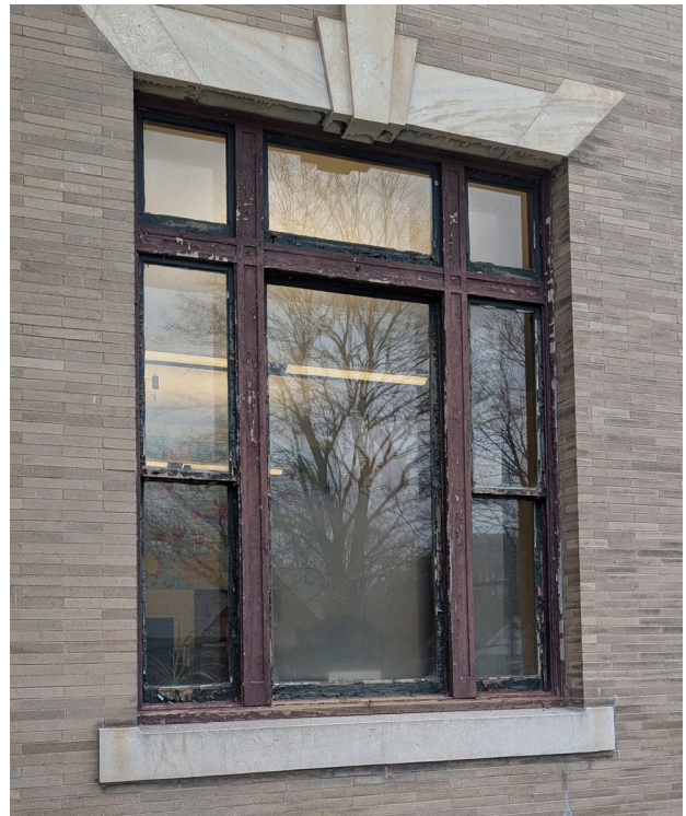
Drafty, peeling windows
