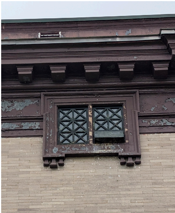
Peeling paint and deteriorated woodwork
